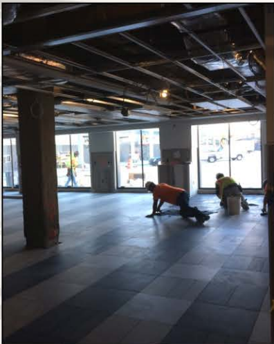
11/16 - Workers continue installing and grouting floor tiles in the Intercity Bus Waiting Area
