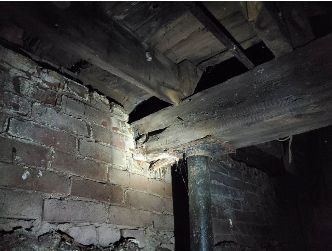
Example of deterioration in wooden structural members where they are in contact with masonry surfaces.
