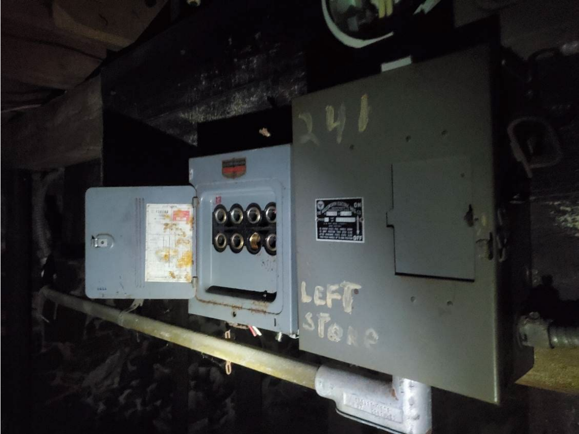
241 Main St, Indian Orchard – Photos showing the current electrical service, meter sockets and fuse boxes, all of which are expected to need replacement.
