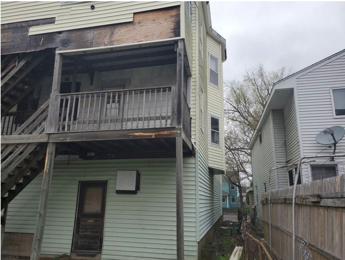
241 Main St, Indian Orchard – Representative photos showing the condition of the rear porch & stair.
