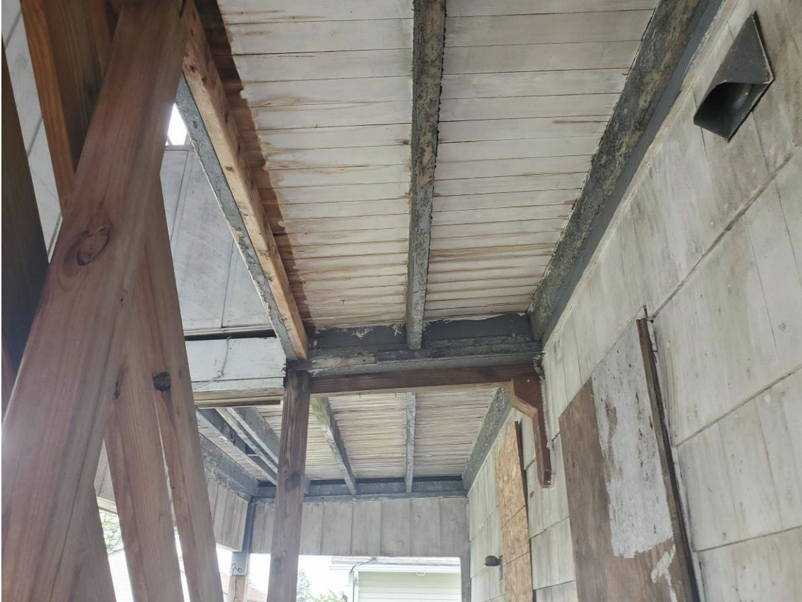
241 Main St, Indian Orchard – Representative photos showing the general condition and varying types of construction used on the rear porch.
