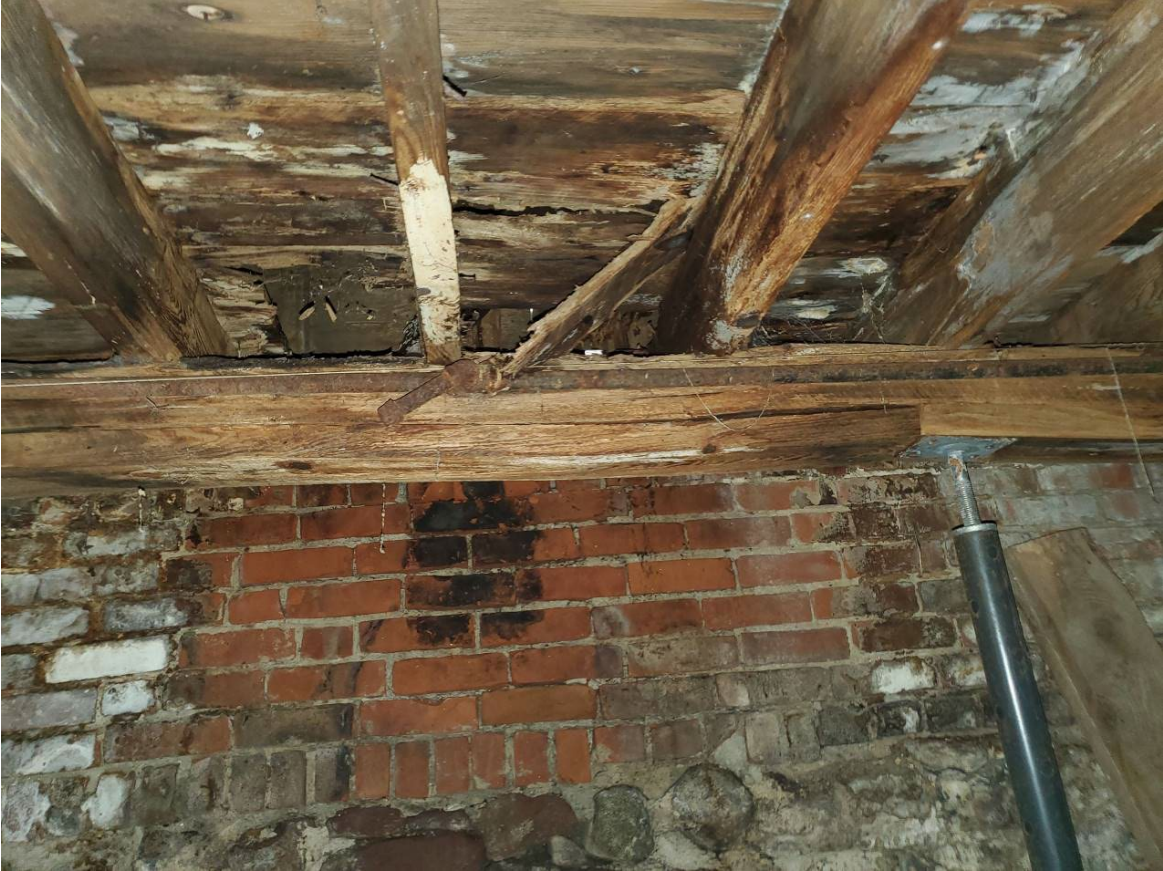
241 Main St, Indian Orchard – Representative photos showing localized water damage in basement (top) and deteriorating floor joists (bottom)
