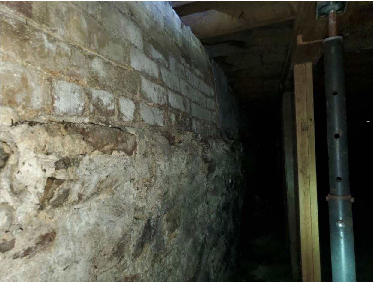
This photo shows the side of the foundation along the driveway that is bowing into the basement.
