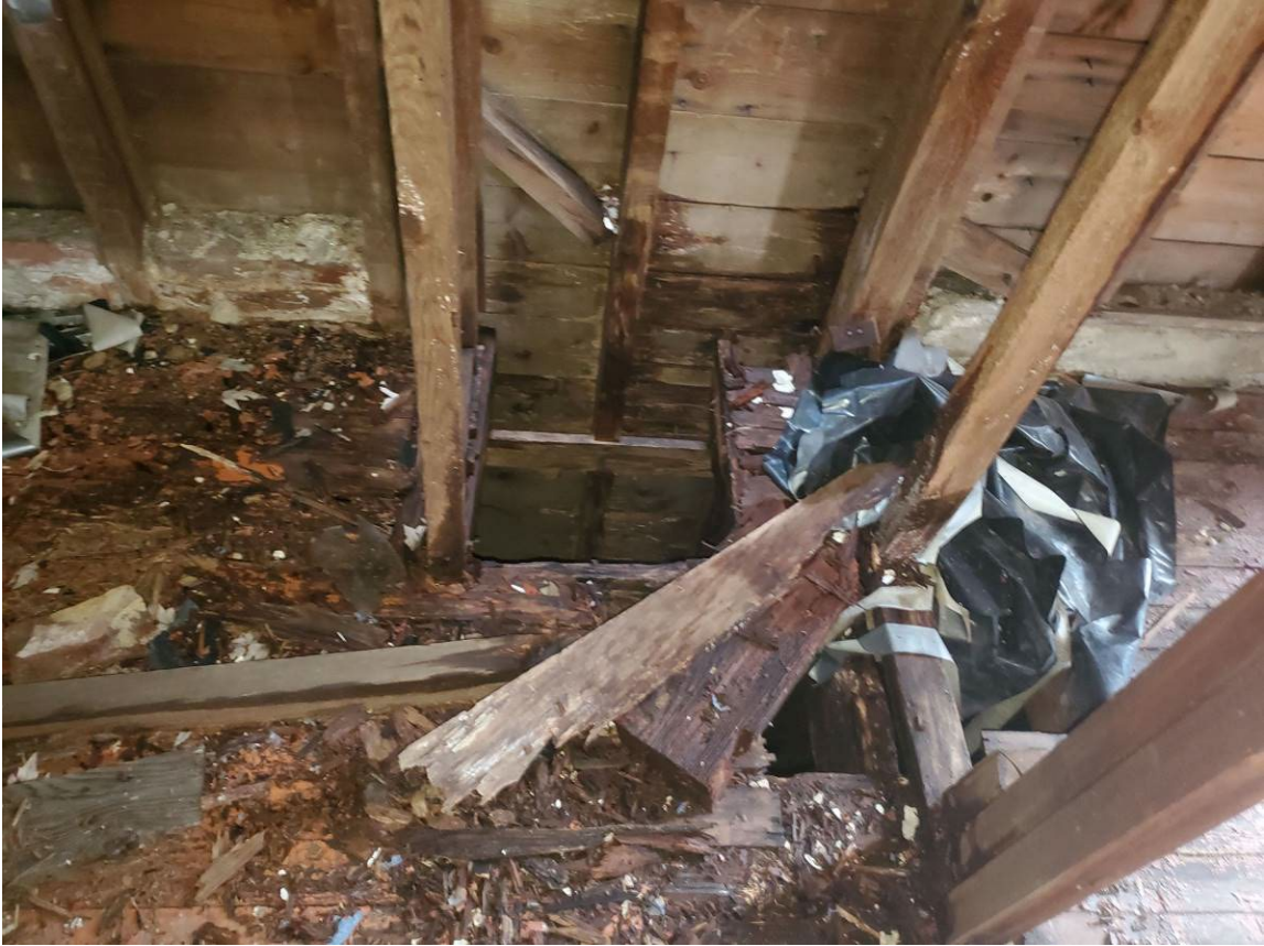
241 Main St, Indian Orchard – Representative photos showing the localized damage from the open chimney hole thorough the roof (top), and characteristic conditions found throughout the upstairs units (bottom).
