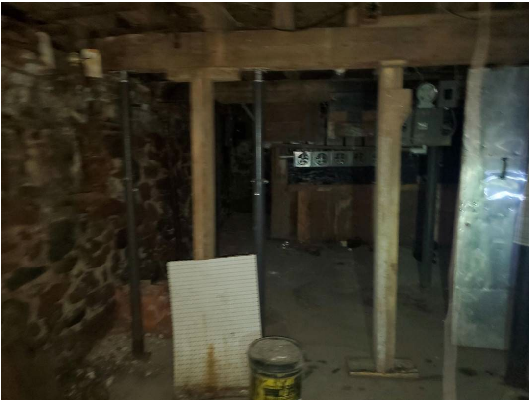
Example of temporary and wooden supports being used as opposed to cement filled steel columns.
