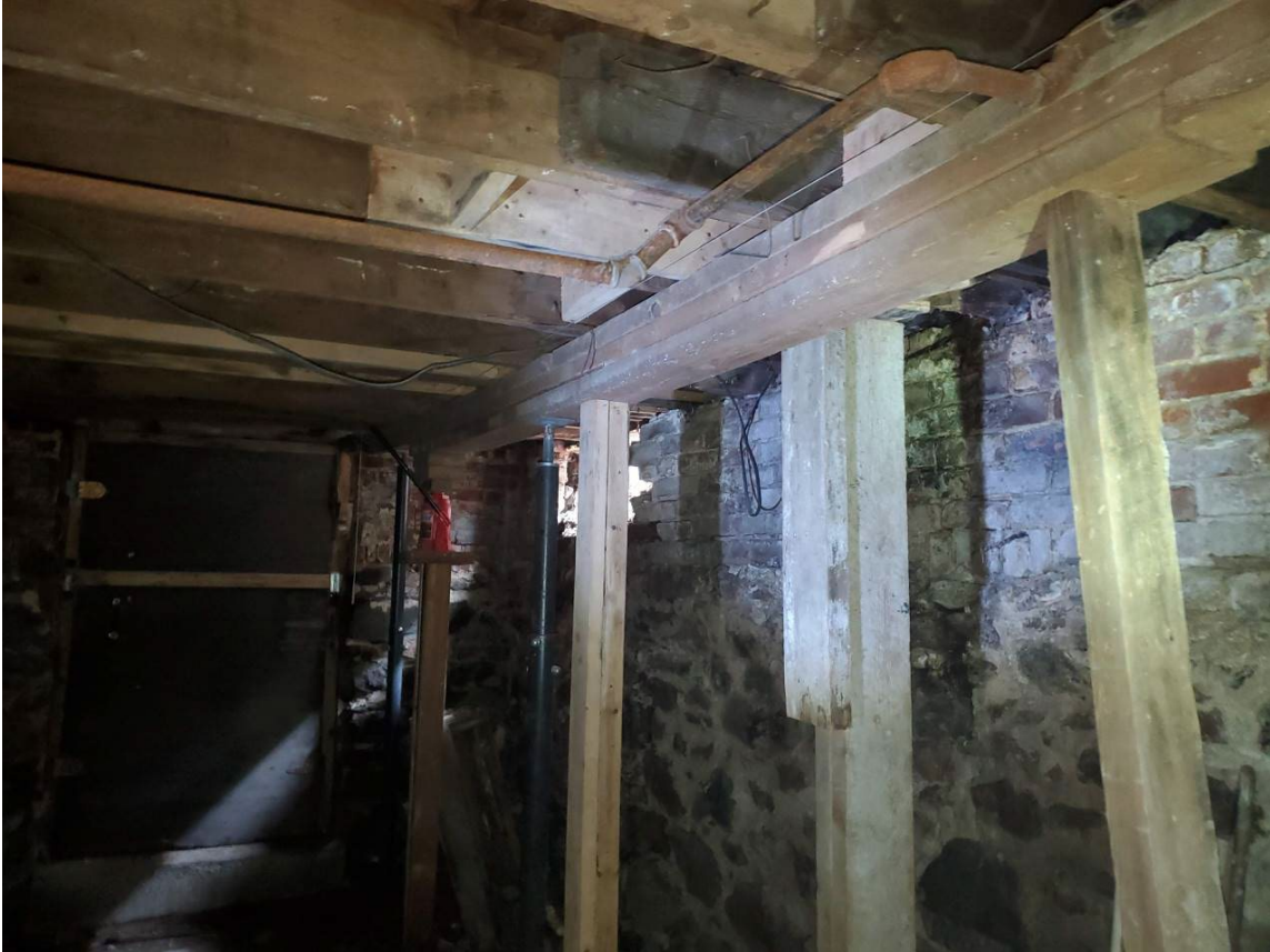
241 Main St, Indian Orchard – Additional photos showing the use of temporary supports and beams in the basement. Some engineering and architectural work is expected to properly evaluate and address.
