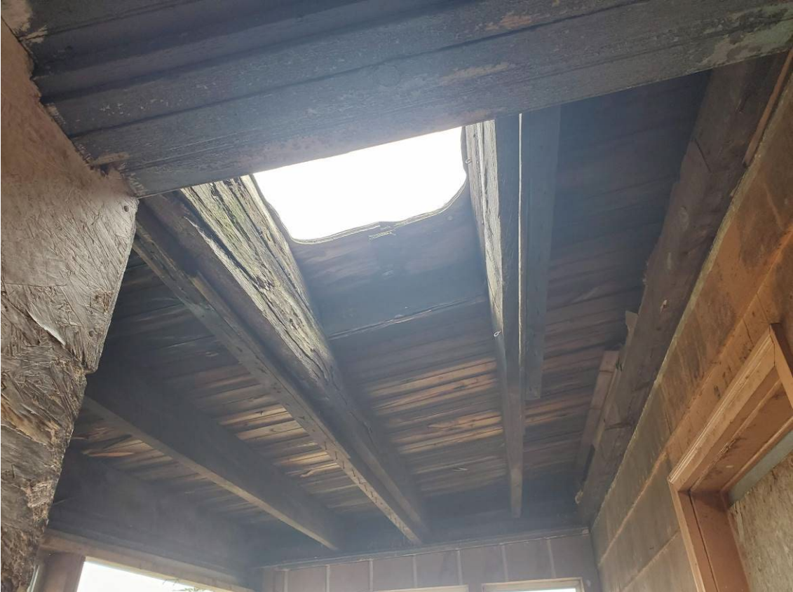
241 Main St, Indian Orchard – Photos showing the open hatchway from the 3 rd floor to the roof (top) and the rot that has been caused below (bottom).
