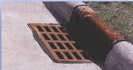
Storm Drain / Catch Basin
