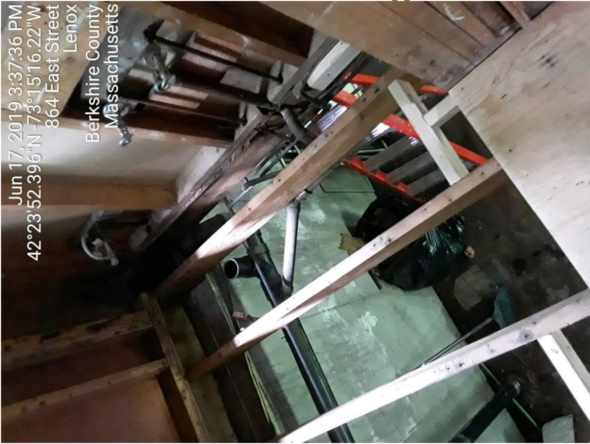
870 East St, Lenox MA – Photo's of bathroom after being gutted and rotten subflooring removed.
