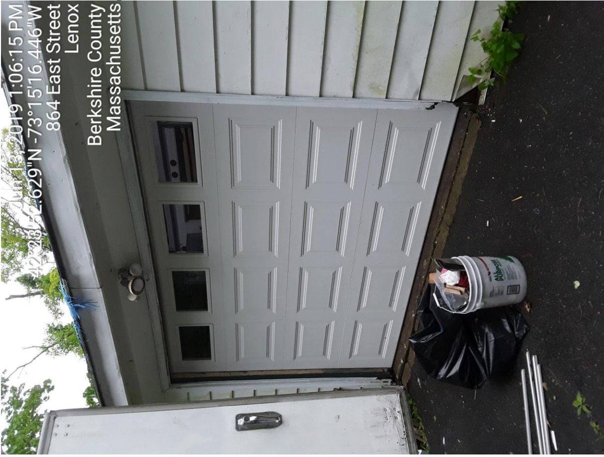
870 East St, Lenox MA – Photos showing new garage door (top) and the garage interior (bottom) after demo and cleanup.
