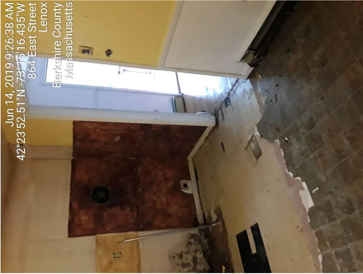
870 East St, Lenox MA – Kitchen with demo in progress (top) and kitchen after completing demo (bottom).
