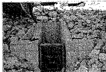
GZA designed this retrofit consisting of an angled slide gate and operator at the MDC Hartford's Reservoir No. 2 in West Hartford, CT
