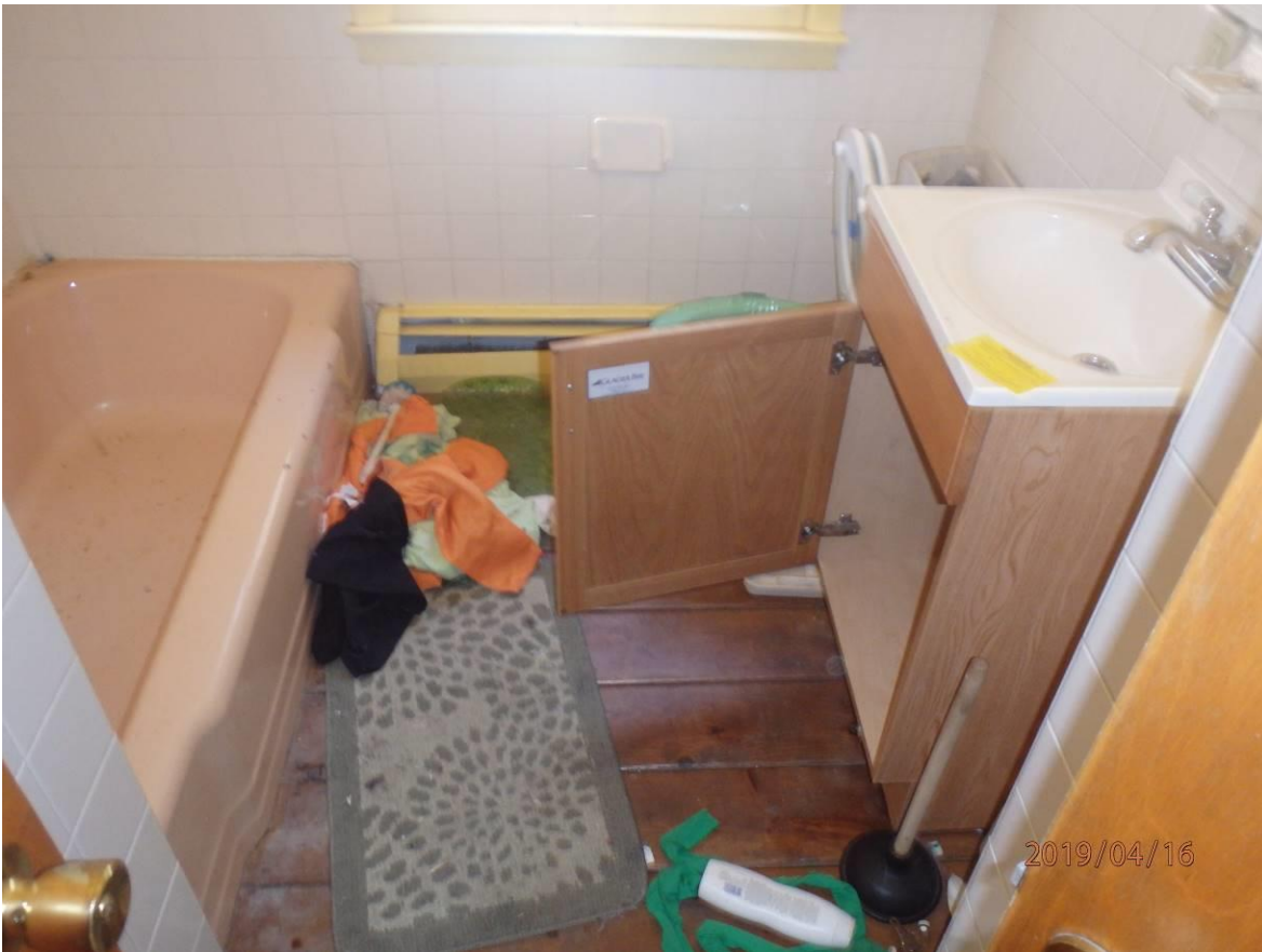
870 East St, Lenox MA –Photos of bathroom with non-impervious wood floor and other damage.
