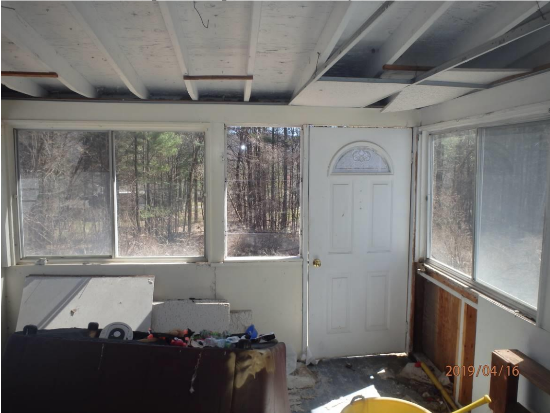
870 East St, Lenox MA – Rear porch (top) where stairs will need to be redone and three season windows removed. The bottom photo is representative of the junk and clutter in the basement.
