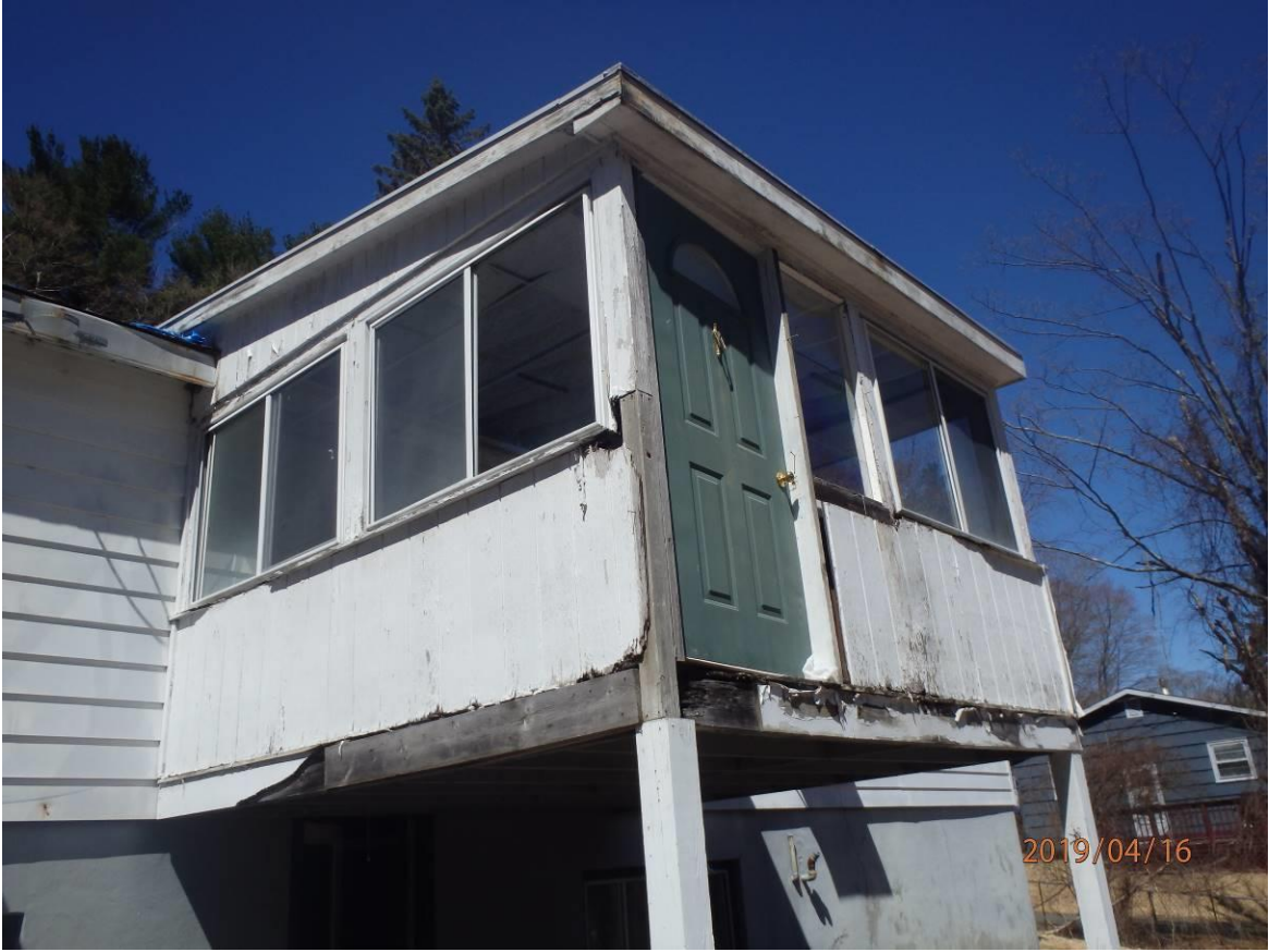
870 East St, Lenox MA – Close up photos of rear porch (top) and garage (bottom). Note how the original garage door was framed in as an effort to create an additional bedroom inside.
