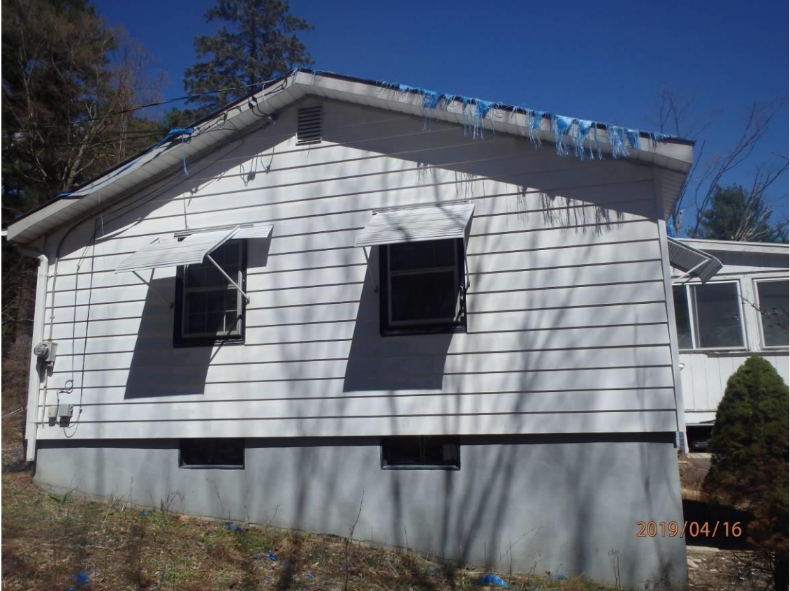
870 East St, Lenox MA Representative exterior photos showing damaged siding, original electrical service (top) and rear porch with rotten wood and missing stairs to ground.
