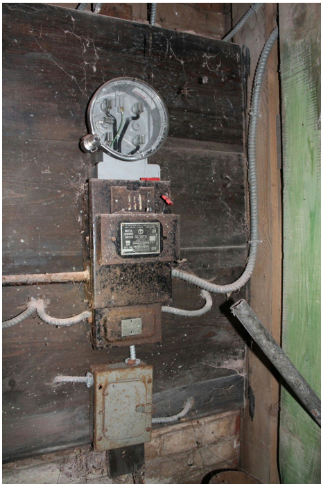
Electrical: See fuses and wiring hazards
