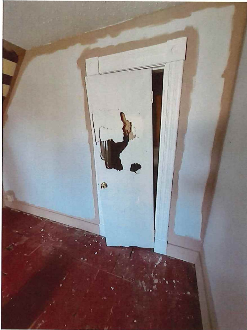
Second and third floor – Replacement of doors. Replace damaged interior hollow core doors
