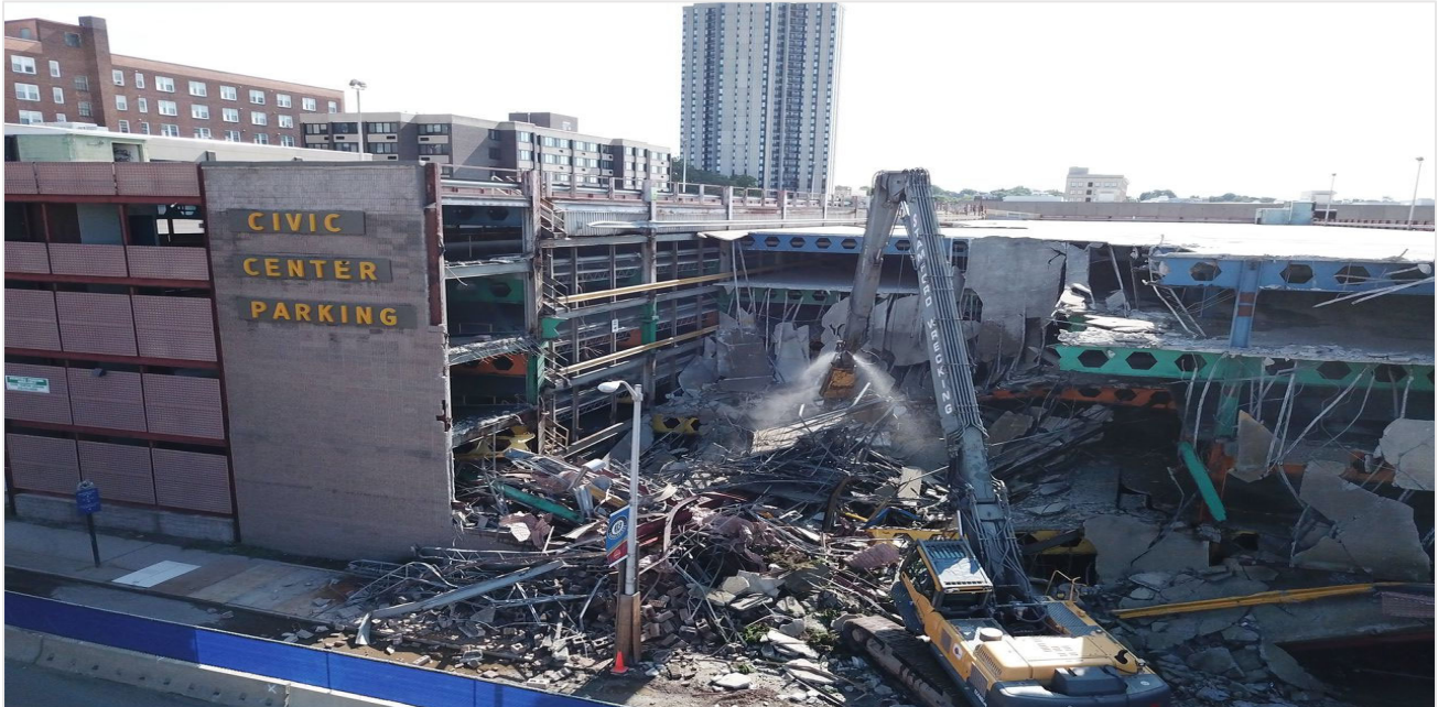
Demolition of Civic Center Parking Garage for new one to be connected to Mass Mutual Center.
